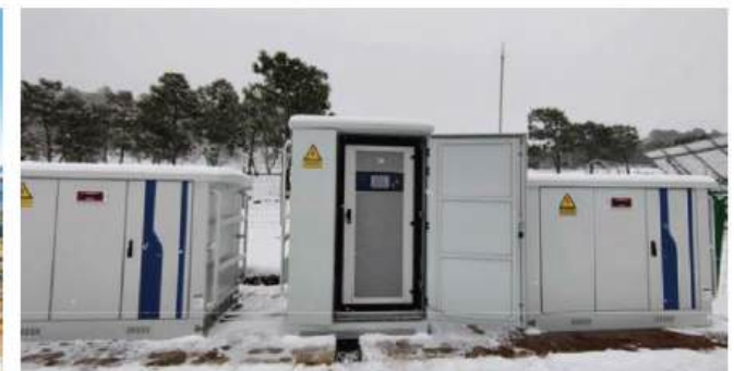
Location: Poland Capacity:250kW/500kWh
